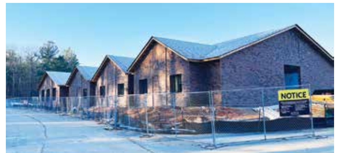
Exterior view of the new wing under construction at the Cassels Health Care Center.
